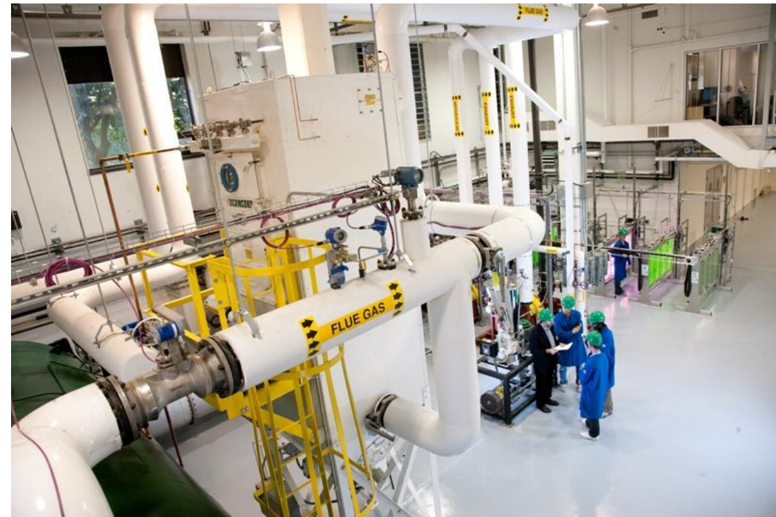
Advanced Coal and Energy Research Facility (1 MWth)
